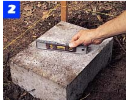
Dig a hole for the first block at the highest point in the grade. Add gravel, install the block, align it with the string, and level it.
