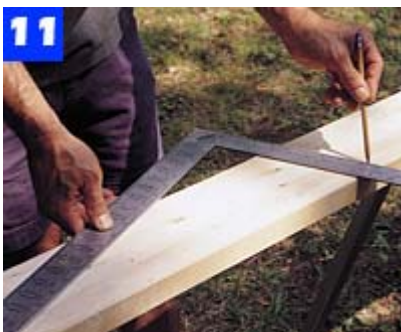
To find the rafter cutting angle, align the 5- and 12-in. marks on the framing square's legs with the edge of the rafter stock.
