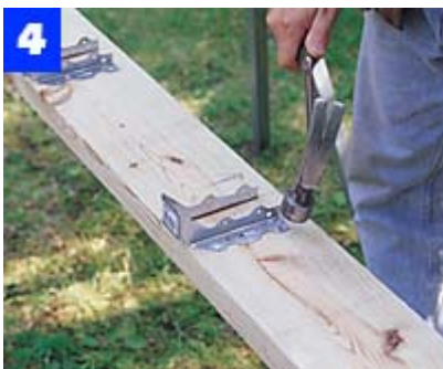
After marking joist locations on long front and rear rim joists, install metal hangers with 1-1/2-in. joist hanger nails.
