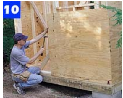
When the framing is in place and the assembly is square and plumb, add the remaining plywood sheathing.
