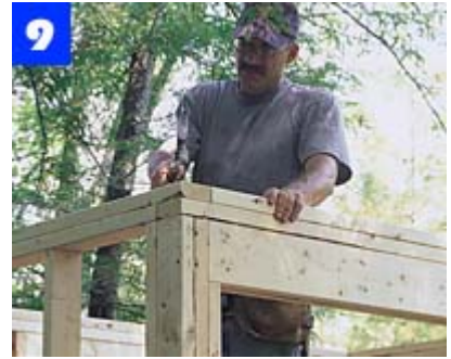
Frame and raise the remaining walls without sheathing. After nailing together the corner studs, add the top plates.
