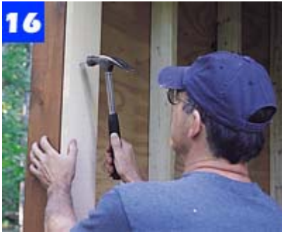
16 Cut stock for doorjamb and nail in place. At a window, install the angled sill piece first, then the top jamb, then side jambs.
